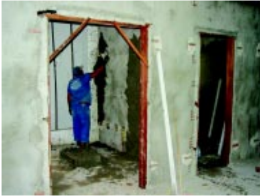
Dengue: obras do Laboratório de Virologia e Terapia Experimental DENGUE: CONSTRUCTION WORK ON THE VIROLOGY AND EXPERIMENTAL THERAPY LABORATORY
